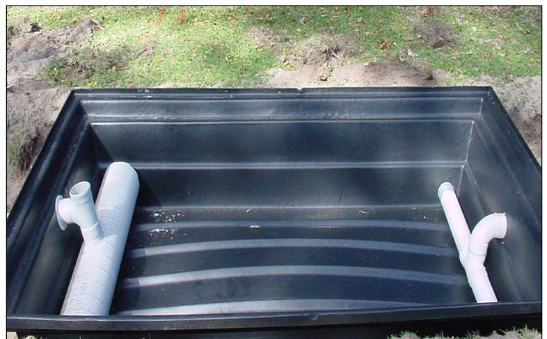
Reedbed plumbing showing inlet T on left and outlet T on right
